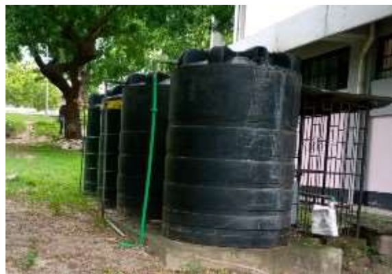
Plate No. 2.3-5: Water Borehole and Storage Tanks at workshop and laboratory construction site.
